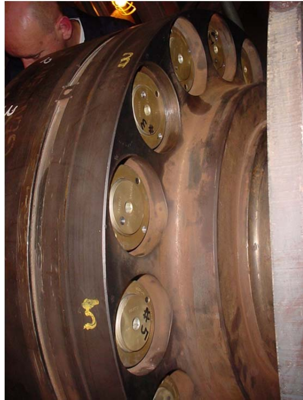
Turbine / Generator Side Photo 2
