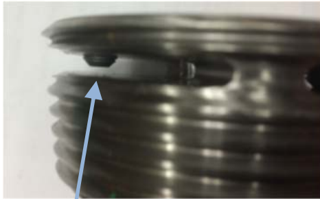
Partially Loose Set screw
